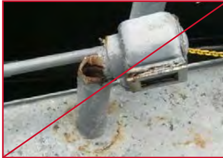
Broken vent pipe that will not pass inspection.
