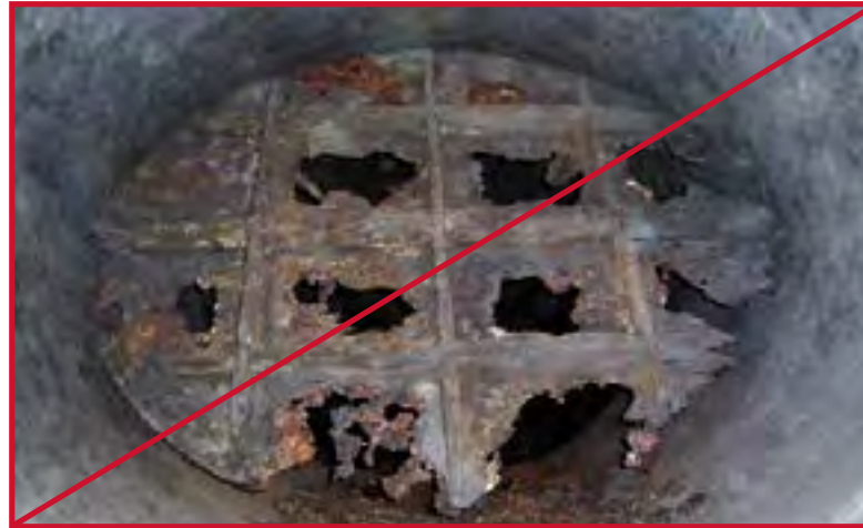
Fire damper that will not pass inspection
