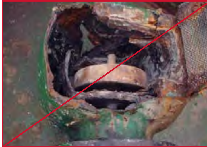
Vent head that will not pass inspection.
